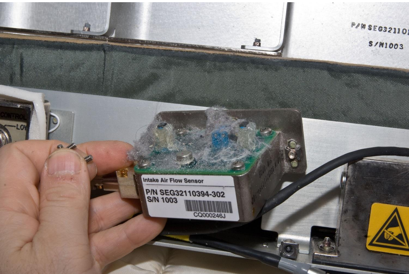
Air flow sensors inside Crew Quarters ducting don't read the correct air velocity when covered with dust.
